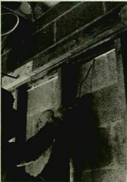
In multifamily work, PEP frequently encounters concrete-block party walls connecting the living space and attic. Warm air rises through the block cores, is cooled in the attic, and falls again. Whether the block is open or closed to the attic, this robs heat from the house and chills the wall. Easily treated in new construction with a course of solid block at the ceiling level, block party walls are a challenge to retrofit. In the photo, PEP cures a related problem—leakage between the party wall and wood framing.
