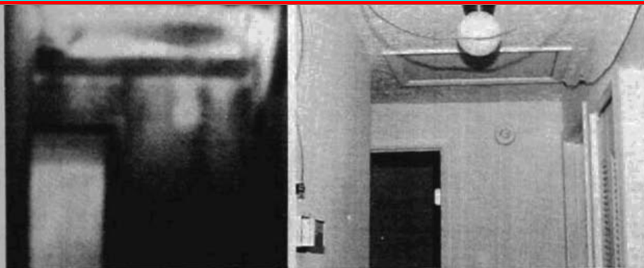
Viewed through an infrared scanner, hot air leaks (light-colored areas) appear around the attic hatch and within the top of the hall-end partition. This thermogram was taken in summer with the house depressurized.
