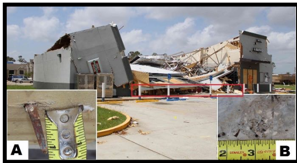
Figure 14. Failure of front (east) wall at this convenience store when the wood frame wall, attached with cut nails. The red box in this image shows where the wall failure initiated. Inset A shows a cut nail protruding from the bottom side of the wall plate. Inset B shows the divot in the concrete slab where the cut nail had been installed.
