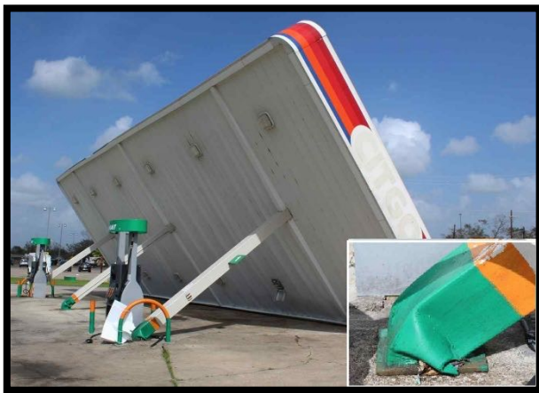
Figure 21. Toppled single column canopy in Vinton, La from strong north winds. The inset image shows plastic hinge formation at the base of the tubular steel column.
