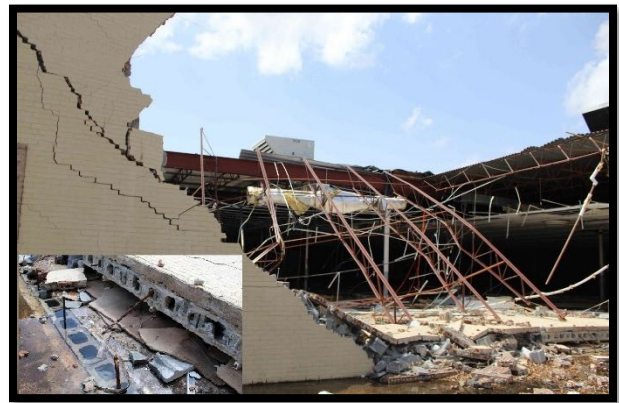
Figure 15. Collapse of the east-facing loadbearing wall on a strip mall. Inset image shows wall and foundation rebar at the base of toppled wall.
