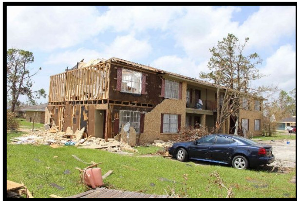
Figure 9. Lost brick masonry on south and east walls along with roof removal on an apartment building on Bancroft Street. The car remained in place.
