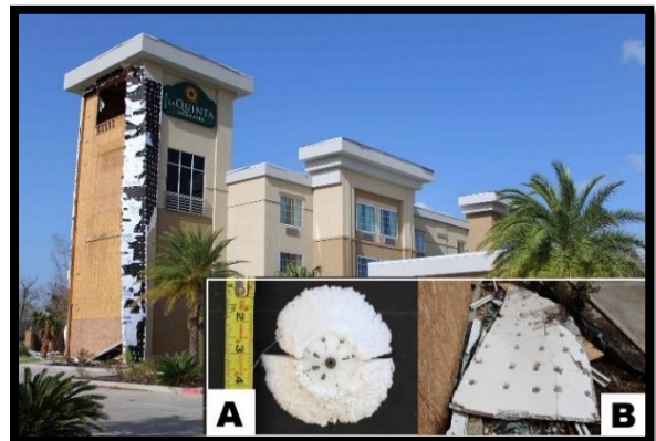
Figure 10. Loss of EIFS cladding from the motel. EIFS panels were secured to OSB sheathing with screws and plastic disks. Inset A shows the cone-shaped area of bead board insulation that remained attached to the walls beneath the fastener plate. Inset B shows the back side of the EIFS panel lying on the ground with holes at attachment points.
