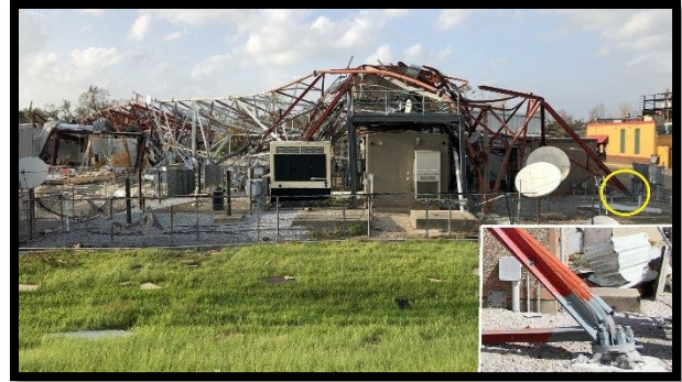
Figure 24. Toppled three-legged tower at KSWL TV in Lake Charles. The inset image is a closer view of the base of the bent leg, inside the yellow circle in the main image.
