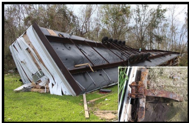
Figure 6. Rolled manufactured home. The inset image shows a severely corroded and broken steel strap, along with corroded anchor head and stabilizer plate.
