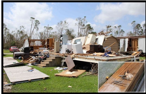
Figure 5. Separation of the wood box from the floor in this manufactured home. Inset image shows wall studs were secured to wall bottom plates with staples and screws, not steel straps as done today.
