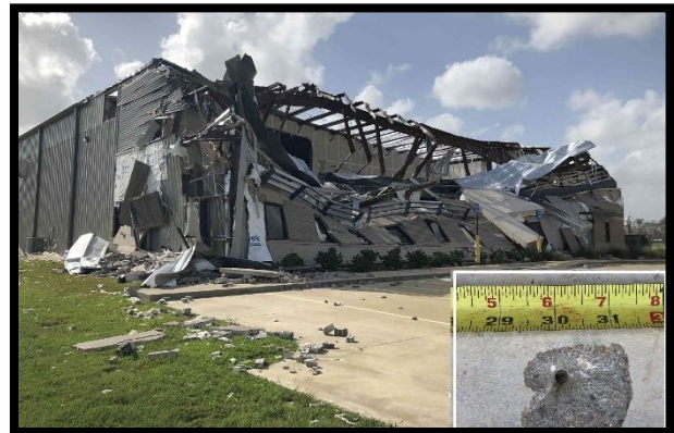
Figure 19. End wall failure on the windward side of this metal building system. The cold formed steel base plate was shot pinned to the concrete foundation and was a connection too weak to resist lateral wind loads.
