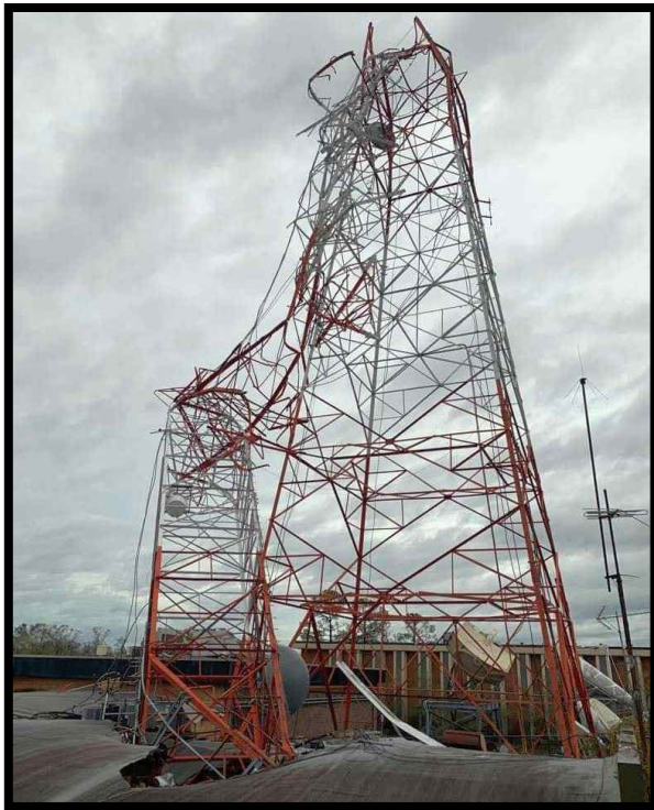
Figure 23. Collapsed four-legged tower at KPLC TV in Lake Charles.
