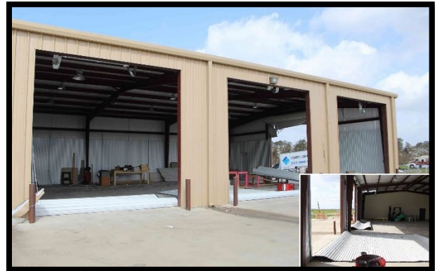
Figure 18. Failure of overhead doors on the windward (east) side of this metal building resulted in outward failure of the north side door. The building frame and cladding remained undamaged. The inset image is a closer view of the failed doors.
