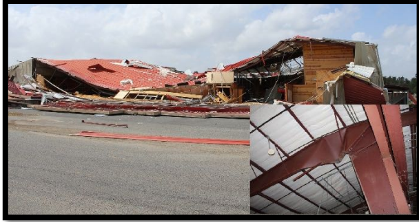
Figure 20. Collapse of a metal building system in Vinton, LA. The north wall blew in, and south wall blew out. The inset image shows plastic hinges developed on the beam (rafter) side of the stiffened beam-column connection.
