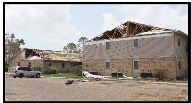
Figure 7. Failure of east facing gable ends on buildings at Fairview Crossing apartments.
