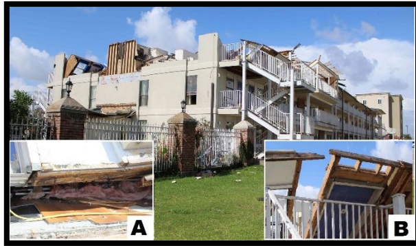
Figure 11. Removal of the roof structure at the east end of the Motel 6. Damage included toppling of top story walls. Inset A shows failed wall bottom plate connections. Inset B shows toppling of the north wall.
