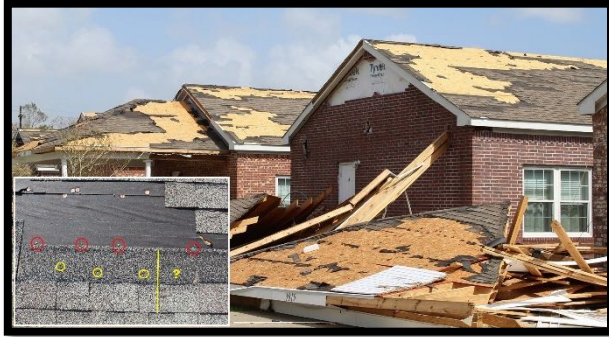
Figure 2. Wind damage to asphalt shingle roof coverings on residences. The inset image shows high nailing (yellow circles) with nails missing top laps in the overlying shingles (red circles).
