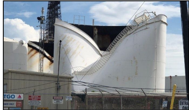
Figure 30. Buckled oil tanks at the Citgo Refinery in Sulphur, LA.
