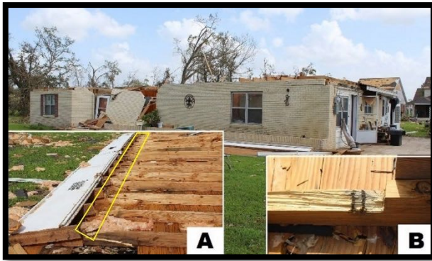
Figure 3. House in Vinton, LA which lost its entire roof. The front side of house faced north and was windward to the strongest winds. Failure of the front doors and windows allowed internal pressure to help lift the roof. Inset image (A) shows upside down roof in the back yard with “birdsmouth” cut outs in rafters (yellow box) and close-up of broken toenailed connection (B) where two parallel rust stains indicate where angled nails had been.
