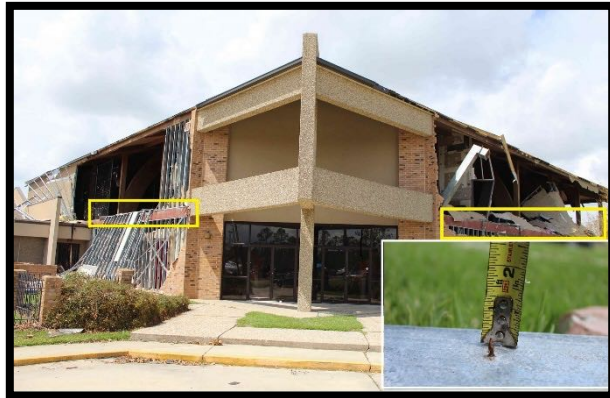
Figure 16. East side of the Glad Tidings church building showing second story wall failures. Cold formed steel bottom plates were nailed into the underlying steel I-beams and simply pulled out of the steel (yellow boxes). The inset image is a close-up view of a protruding nail in the upside-down wall bottom plate.
