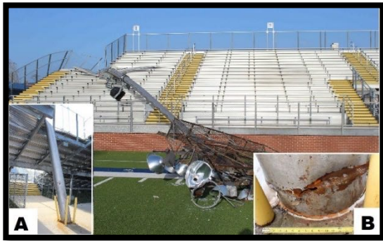
Figure 26. Topped tapered steel light poles at the high school stadium in Sulphur, LA. Poles buckled at their bases then bent again when hitting the stands (inset A). Close examination of the pole bases revealed corrosion (inset B).
