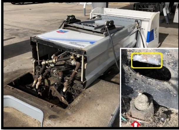
Figure 28. A toppled gasoline pump. The inset image shows a close-up of the bolted connection at the base of the pump. Note the slight downward deformation in the steel angle (yellow circle) and slight upward deformation in the steel washer (red arrow).
