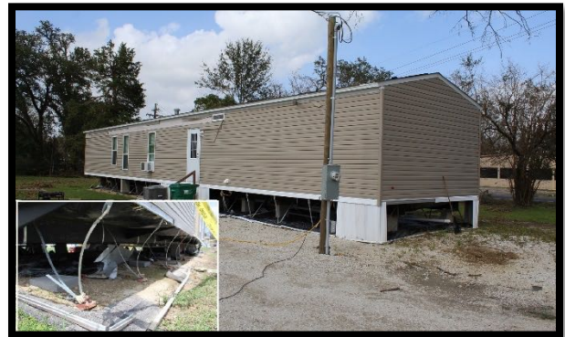
Figure 4. Damage to a newer manufactured home with over-the-top and frame ties included loss of skirting, siding, and roofing. The inset image shows slackened ties, apparently due to rocking movement of the home during the hurricane.
