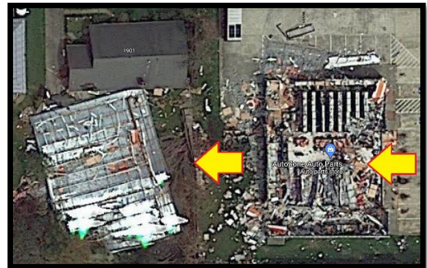
Figure 13. Aerial image showing complete removal and flipping of the Auto Zone roof into a neighboring back yard due to internal pressure effects after front window failure. Note the lack of damage to the house. Source: Google.
