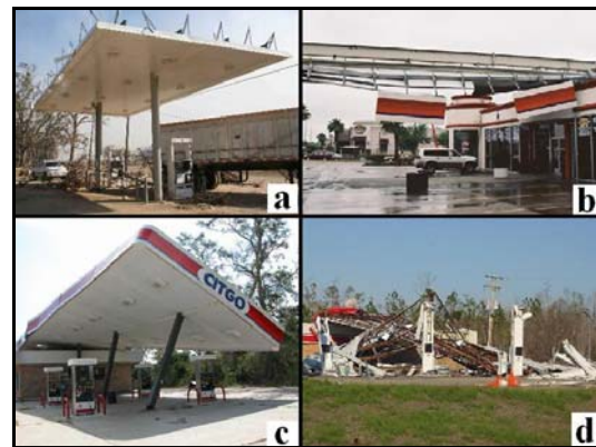
Figure 2. Degrees of wind damage to gas station canopies in Hurricane Katrina: a) loss of fascia (DOD 2), b) metal panels stripped from canopy (DOD 3), c) rotation of columns (DOD 4), and d) collapse of canopy (DOD 5).
