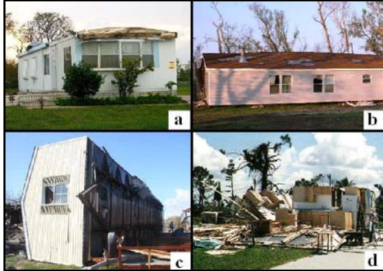
Figure 5. Various DODs to manufactured homes: a) loss of the roof covering (DOD 2), b) sliding of unit off its piers (DOD 3), c) rolling of home (DOD 5), and destruction of roof and walls leaving the floor in place (DOD 6).
