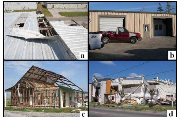
Figure 11. Various DODs to metal buildings in Hurricane Katrina: a) the threshold of visible damage (DOD 1), b) failure of overhead doors (DOD 2), c) loss of metal roof and wall panels (DOD 3), and d) failure of the windward end bay leading to rotation of the columns (DOD 4) and buckling of roof purlins (DOD 5).
