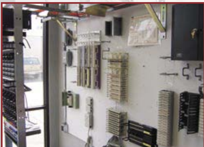
Figure Five: Equipment-mounted backboard.
