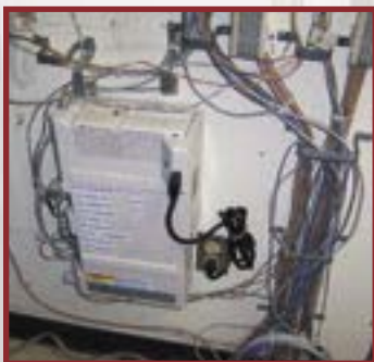
Figures Three And Four: Telecom room/closet backboard and mount height.
