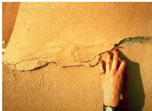
A waterproof coating is an inappropriate substitute material to apply to adobe as it seals in moisture and may result in spalling. Photo: NPS files.
