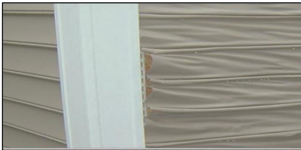
Figure 2. Vinyl Siding Distortion
