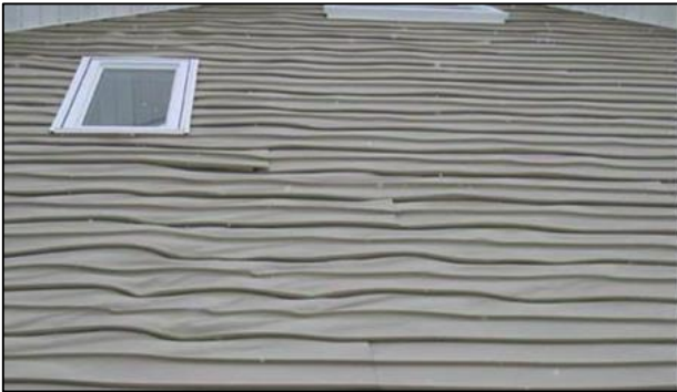
Figure 9. Opposite Wall Distortion
