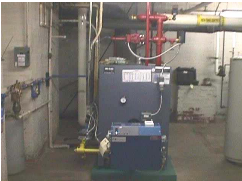
Photo of a newly installed boiler, Sept-2005. This is a 787,000 BTU input cast iron, Weil McLain boiler, equipped with a Power Flame burner.
