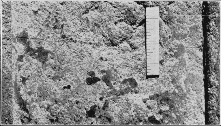
FIGURE 4.—Concrete surfaced with 1:3 cement mortar.
