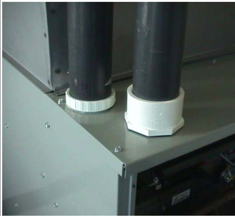
Figure 25: Exhaust Vent / Combustion Air Intake
