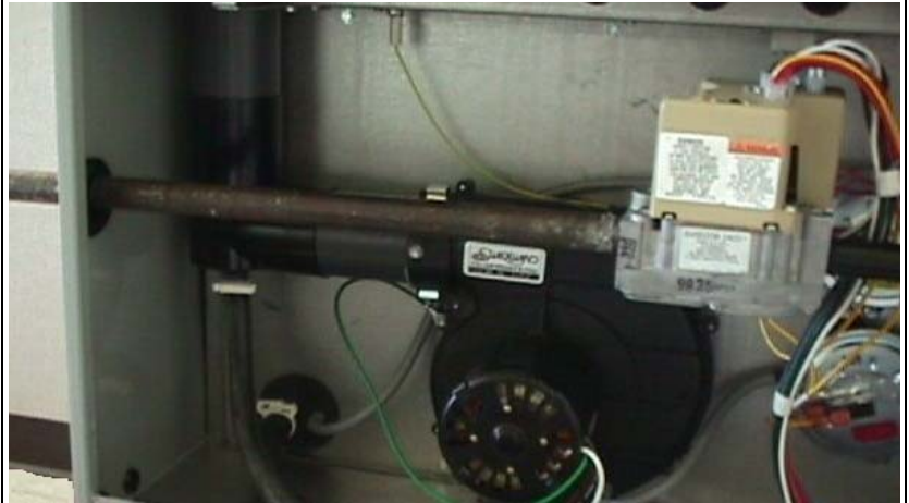
Figure 29: Furnace Gas Pipe Connections - Note Rubber Grommet
