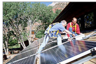
Periodic visual inspection may be necessary to properly maintain your solar system. Photo credit: Robb Williamson.
