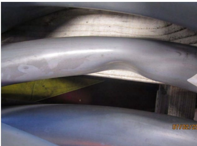
Figure 3. Defect: Large Dent
