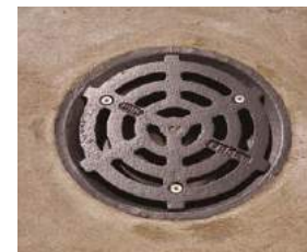
Ductile iron circular grating in a concrete floor
