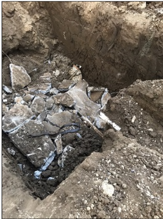
Cracked tank bottom. In this picture, the tank side(s) have been removed.
