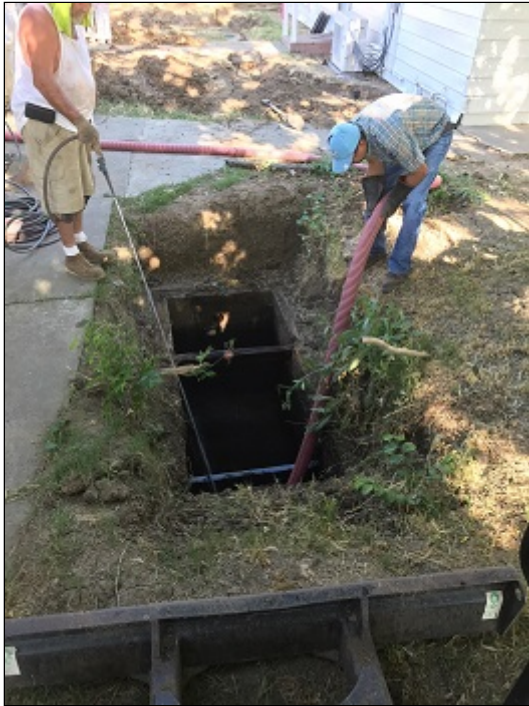
Registered Septic Tank Pumpers pumping a tank. Notice the pressurized water hose used to knock down all solids for pumping.
