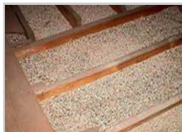
Vermiculite insulation between attic joists; click to view larger version of image
