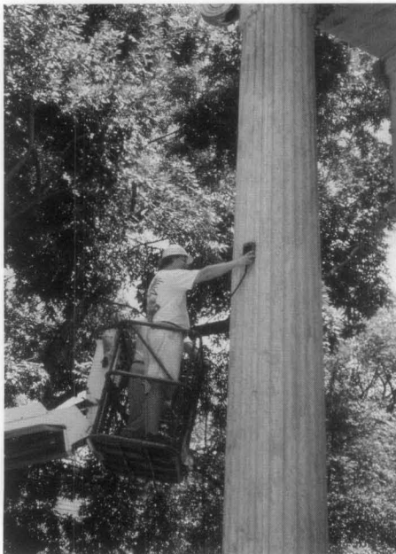
Fig. 11. Impulse radar is being used to evaluate both the orientation and depth of cracks visible on the surface of the column shaft. Photo: Edmund P. Meade, P.E.
