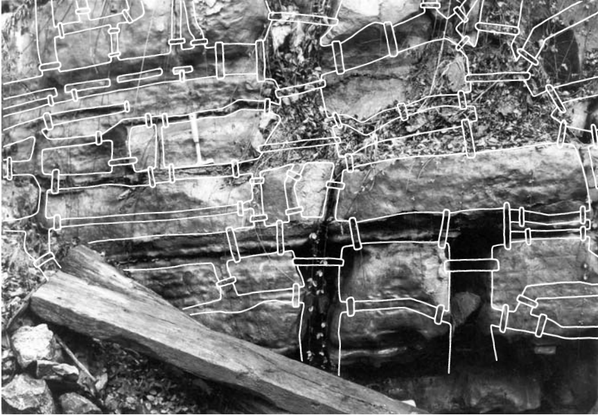
Figure 6. Fractures behave as though they were pipes in limestone bedrock and convey water to the water table.
