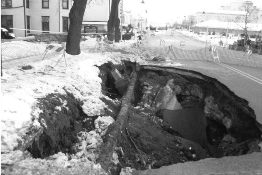
Figure 12. This sinkhole in Dauphin County has exposed a utility pipeline.
