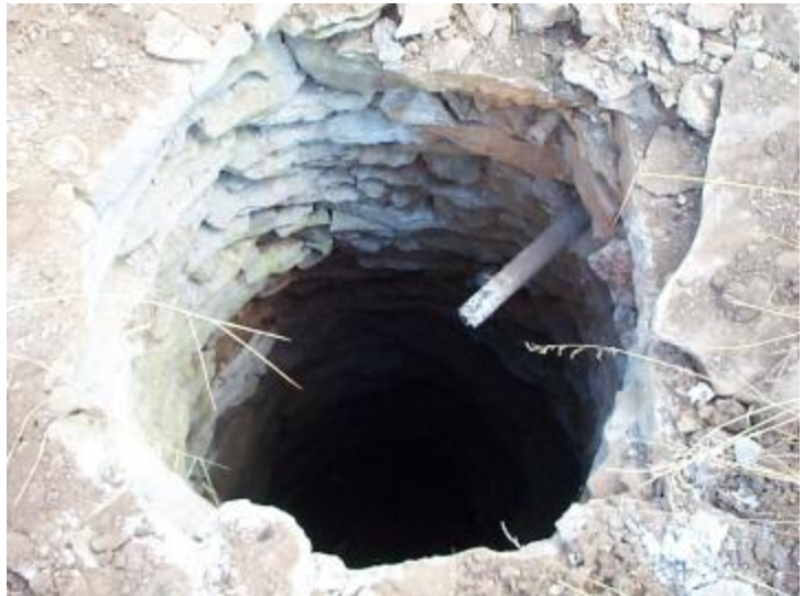
Hand-dug wells that have been abandoned need to be plugged to protect human health and safety.
