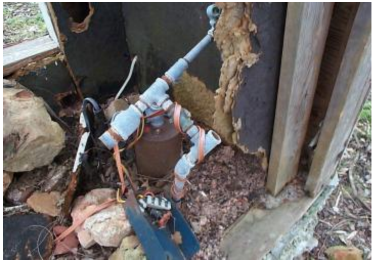
Sometimes, wells are enclosed in a well house.
