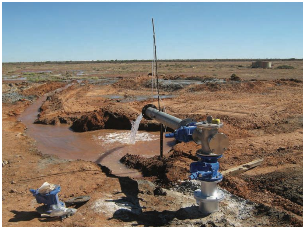
Flowing artesian bore (prior to site cleanup)
