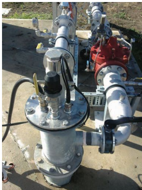
Two views of headworks on an injection/extraction bore
