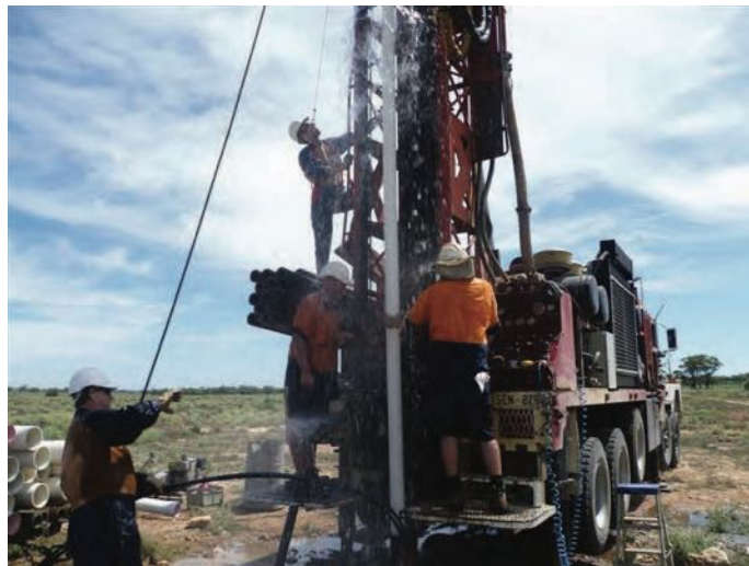
Running casing into the hole Photo courtesy of Kangarilla Drilling Pty Ltd.
