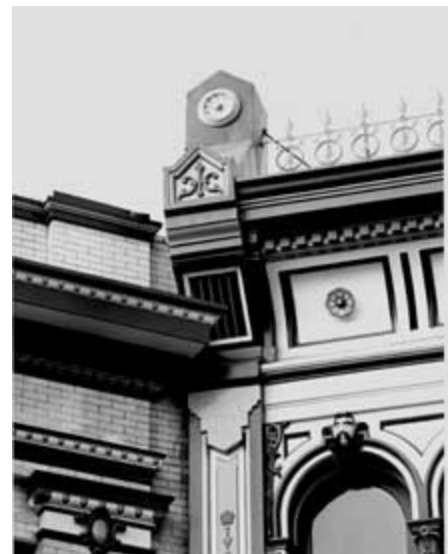
This shows a detail of a polychromed cast-iron facade in Petaluma, California, 1886 (O'Connell and Lewis, Architectural Iron Works, San Francisco). Photo: Don Meacham.
