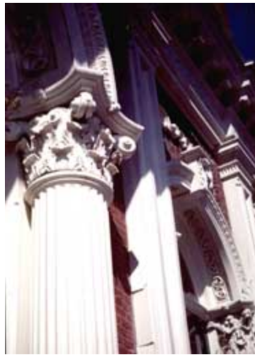
Fiberglass columns and aluminum capitals were installed to replicate the ornamental features on the east facade of the New Market Theater in Portland, Oregon. Photo: William J. Hawkins, III.
