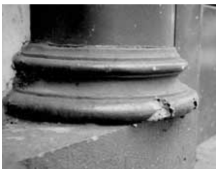
This lightweight fiberglass column at street level sustained damage from impact within a few years of installation. Photo: Building Conservation Associates.
