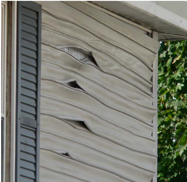
Figure 1a. Vinyl siding with extreme permanent distortion
