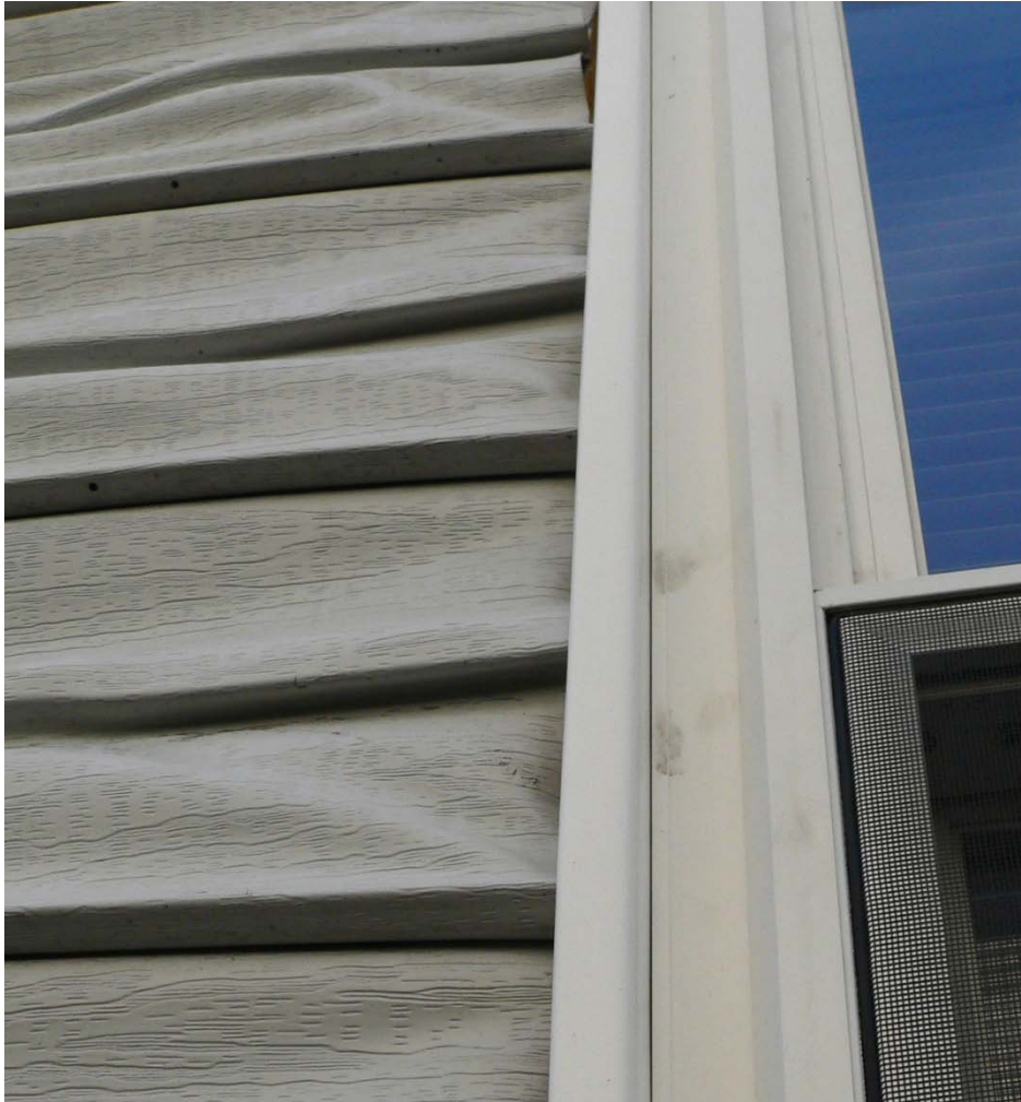
Figure 7. Permanently distorted vinyl siding adjacent to an undistorted vinyl window frame
