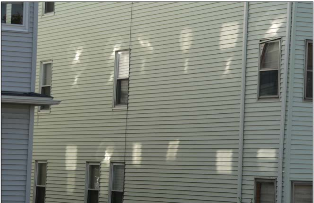
Figure 13. Image of varying IGU reflection shapes from a series of double-hung windows on a house that is ~30 ft. away and parallel to the reflecting glass surfaces
