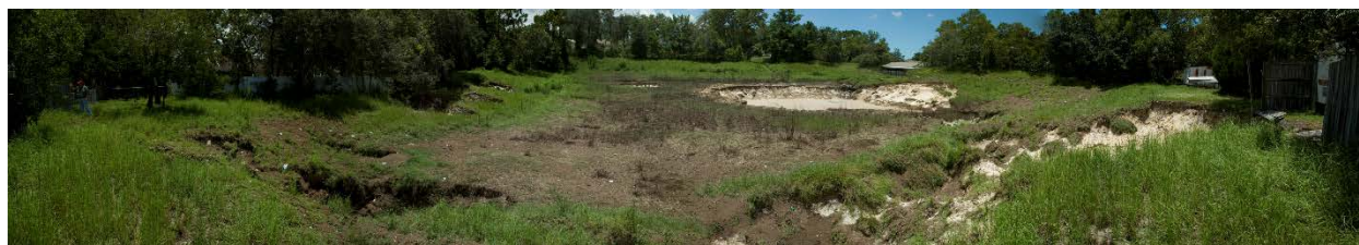
Figure 5. Sinkholes formed within and near this stormwater pond after Tropical Storm (TS) Debby in June 2012 in Spring Hill, Hernando County.
